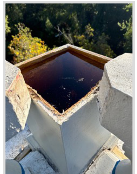
Inside the railing, untreated
