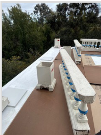
Each piece of the decorative roof railing had to be numbered for de- and re-installation
