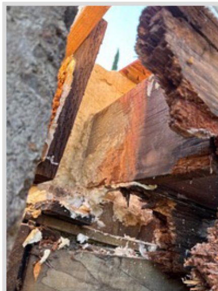
Wood crumbling from water damage
